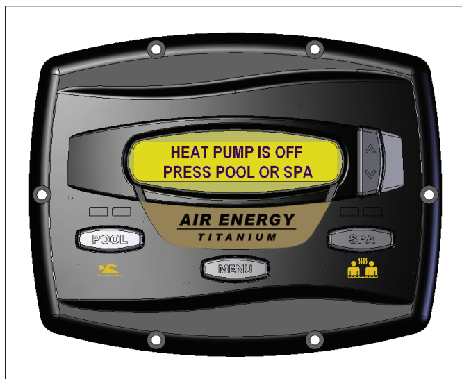
Figura 18. Panel de Control Principal
